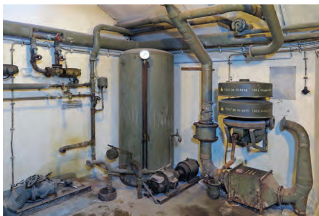
Original ventilation, filtration and other equipment in the Kaufmann Bunker
